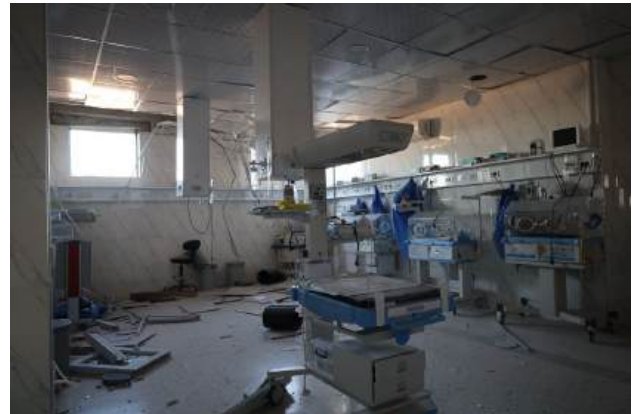
A section of the damage at Ibn Sina Children's Hospital in Idlib
